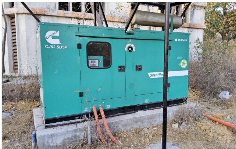
Figure 4 Existing DG Set Inside the Campus
