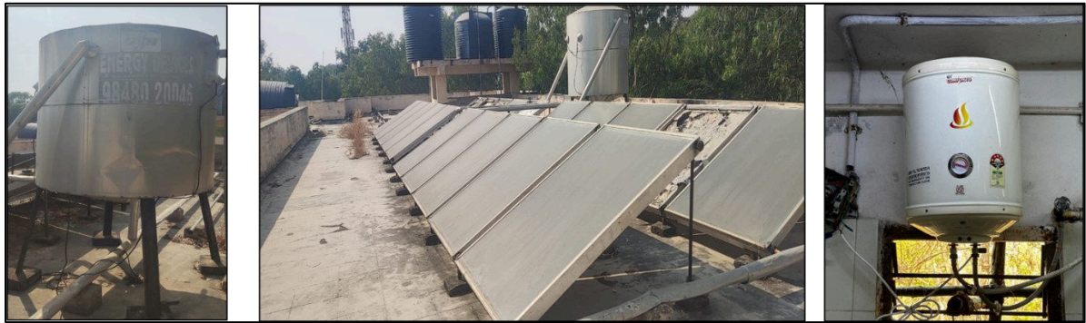
Figure 27 Existing Conditions of Water Heating Systems in Hostels
